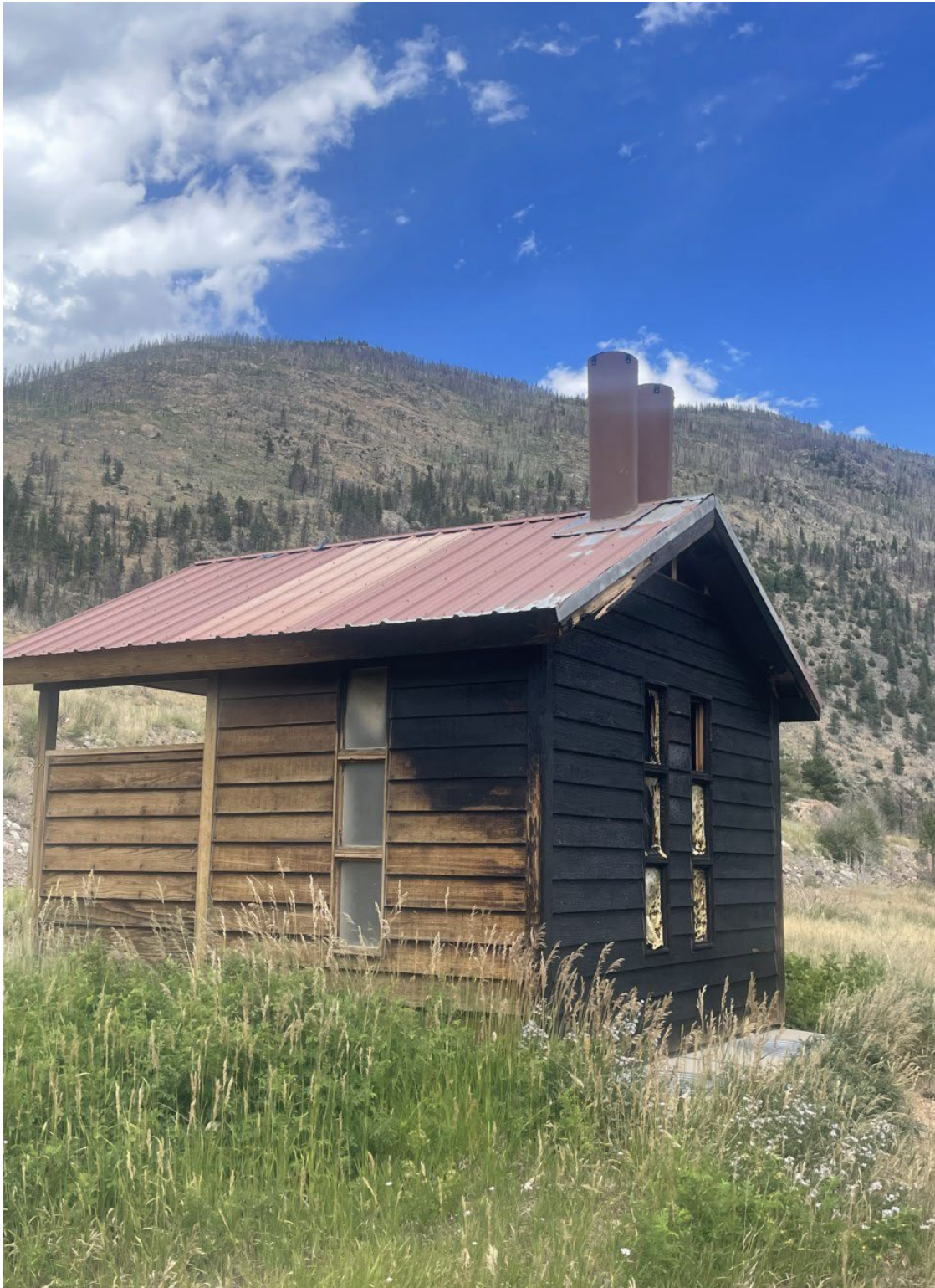
Tunnel Picnic Area toilet damage
